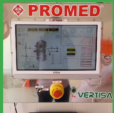
PROMED CONTROL PANEL
