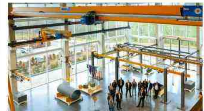
On 3 levels, different crane systems are waiting to be tested at length by visitors like you.
